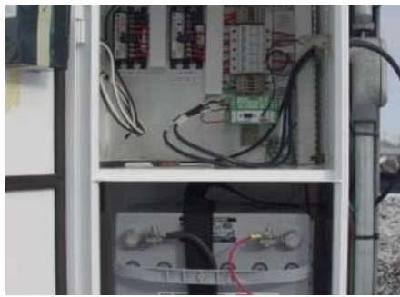
Solar Interference System (SIS) from Phoenix Contact provides wireless telemetry at remote tank monitoring site without an A.C. power source
