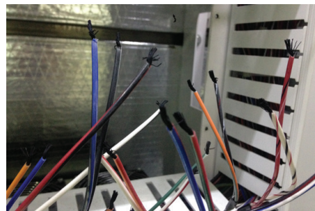
Figure 3. Corroded wires inside of an enclosure from condensation and corrosion problems.
