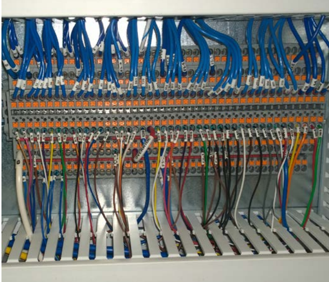
Figure 2: With the 1.5-mm terminals, Forpak saves at least 20 percent on the terminal space needed for sensors and servo encoder cables, and sometimes as much as 35 percent.
