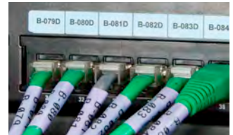
Patch Panel Labels
