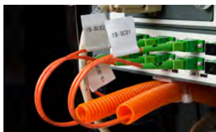
Fiber Optic Cable Markers
