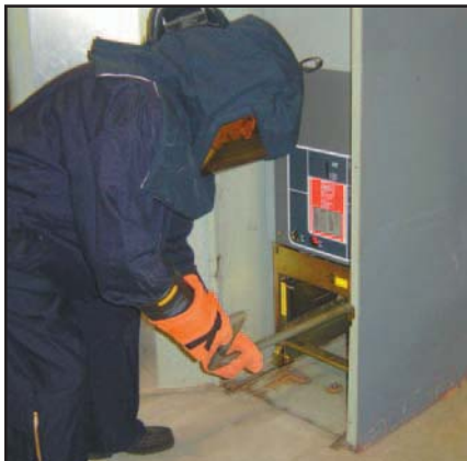
Personal Protective Equipment Required for ARC Flash Exposure
